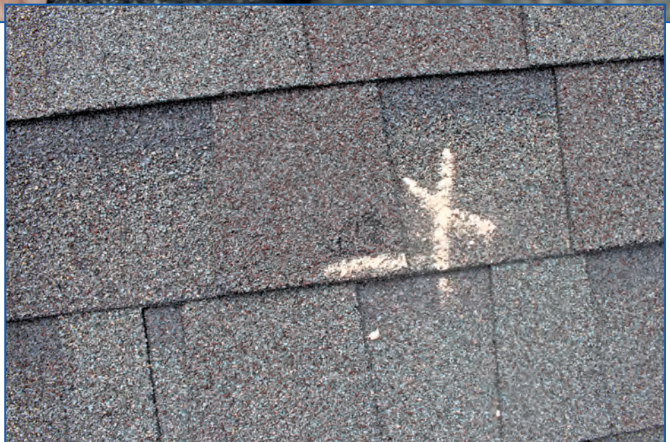
Figure 1 – Example of a hail-caused bruise looking down at the top of an asphalt shingle.
