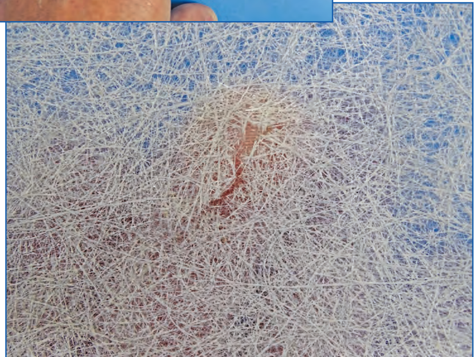
Figure 14 – Close-up of fracture in reinforcement shown in Figure 13.
