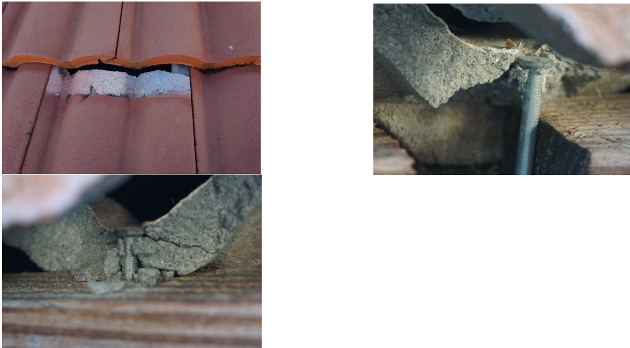
Figure 2: Fracture through the fastener hole caused by overdriven fasteners
