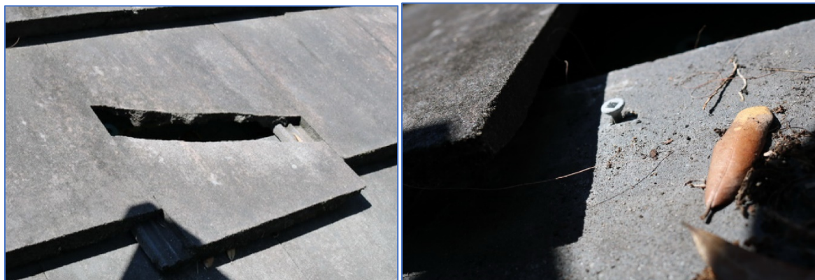
Figure 3: Tile fracture caused by an elevated underlying fastener
