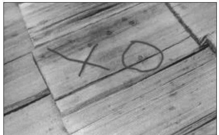
Figure 6. Hail-caused split in a cedar shake with the impact mark circled.
