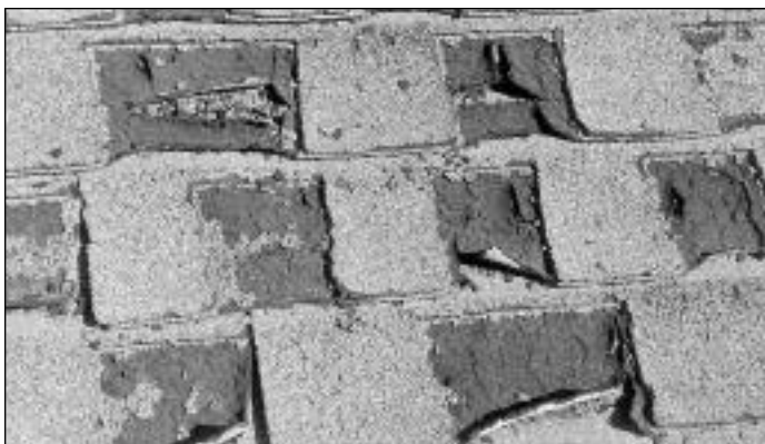
Figure 5. Delamination and flaking of the tack coat and granules because of material deficiencies.
